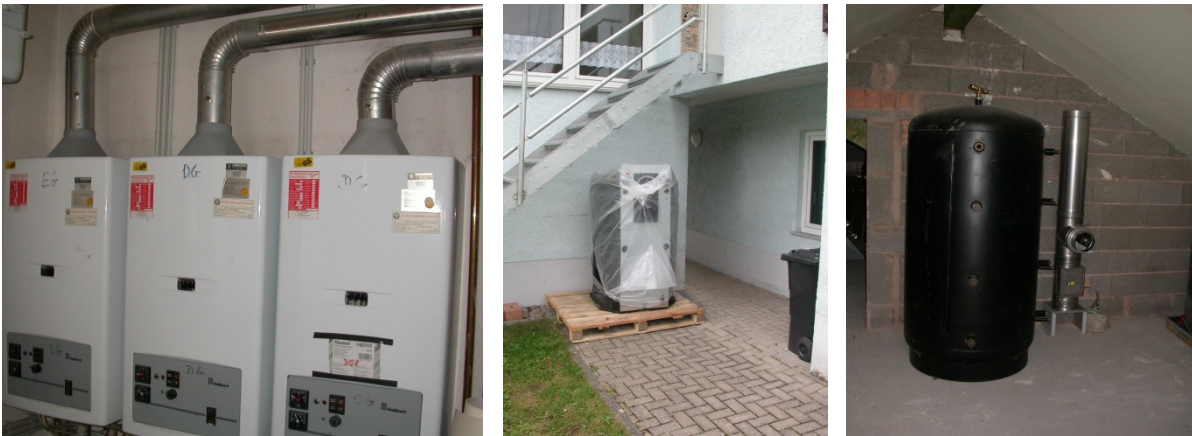
Figure 3: Example for the formerly gas heater, site photos from the building phase
